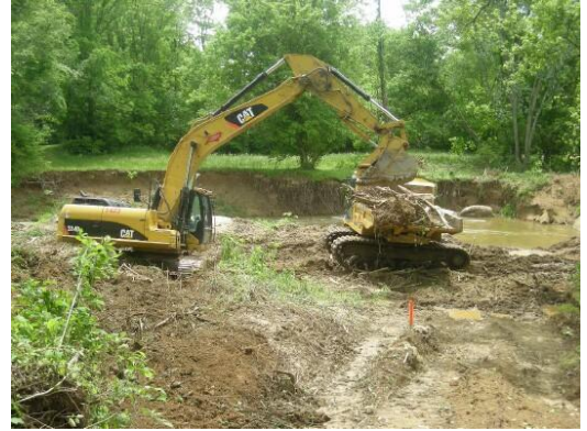
Work being done to restore the Ararat River in Mount Airy. This section will be available for Delayed Harvest (DH) fishing starting in October 2011
