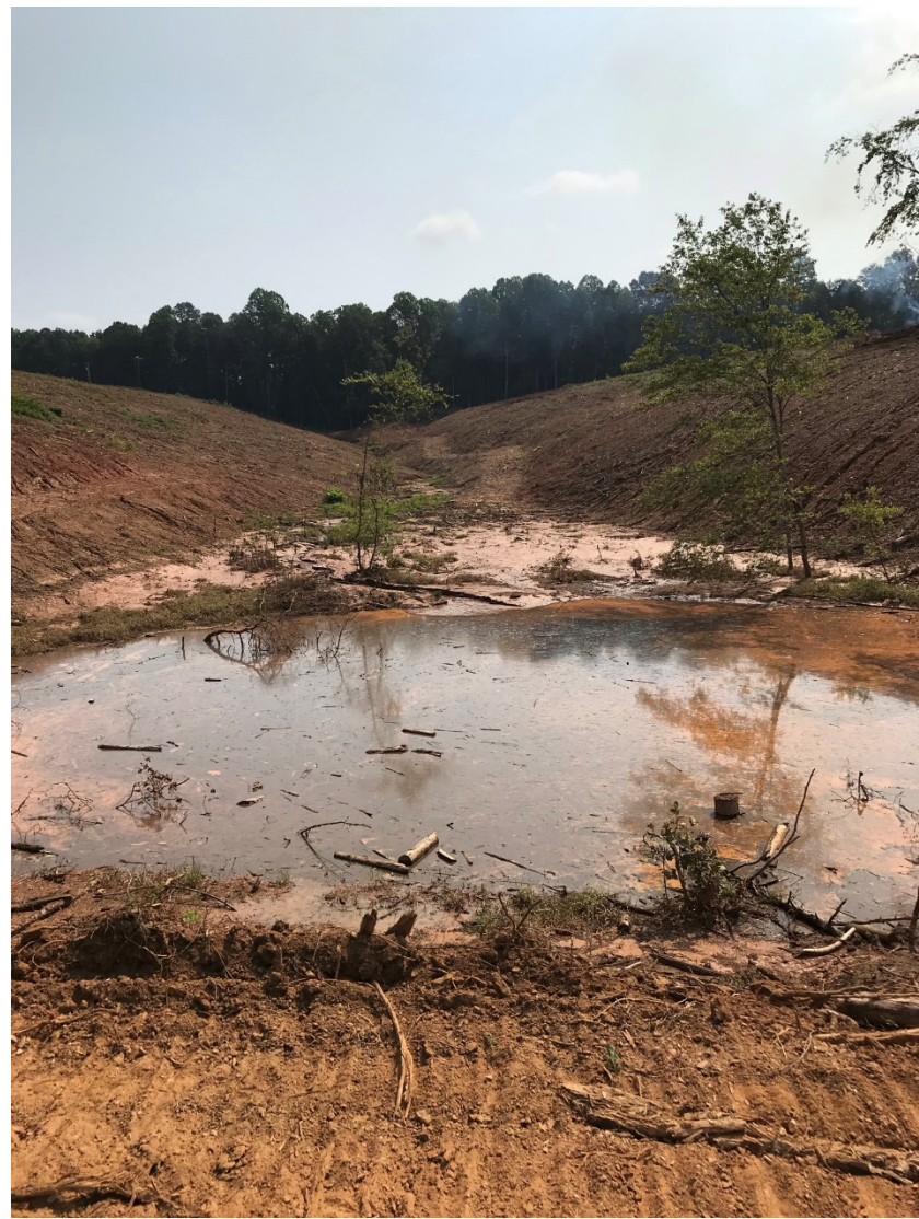
Photo 4: Significant sediment deposit within pond
